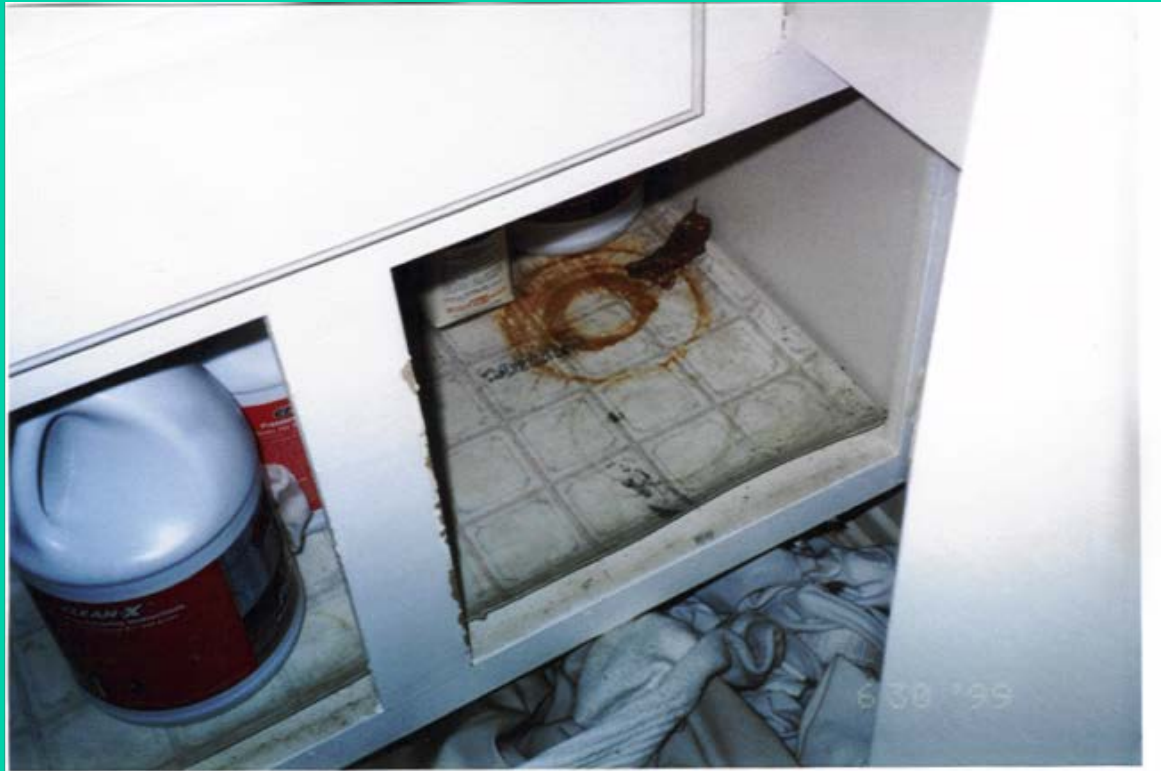
Master bathroom sink with staining
