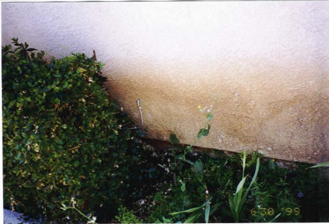
Conduit and hole in wall outside of the family room side of residence
