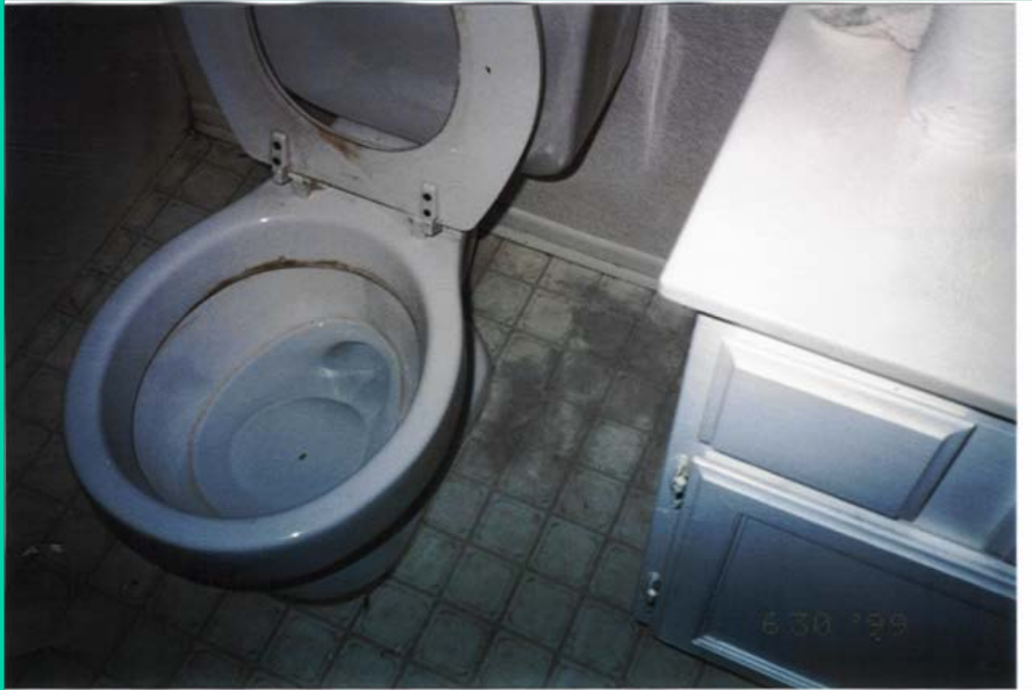
Master bathroom with staining on linoleum
