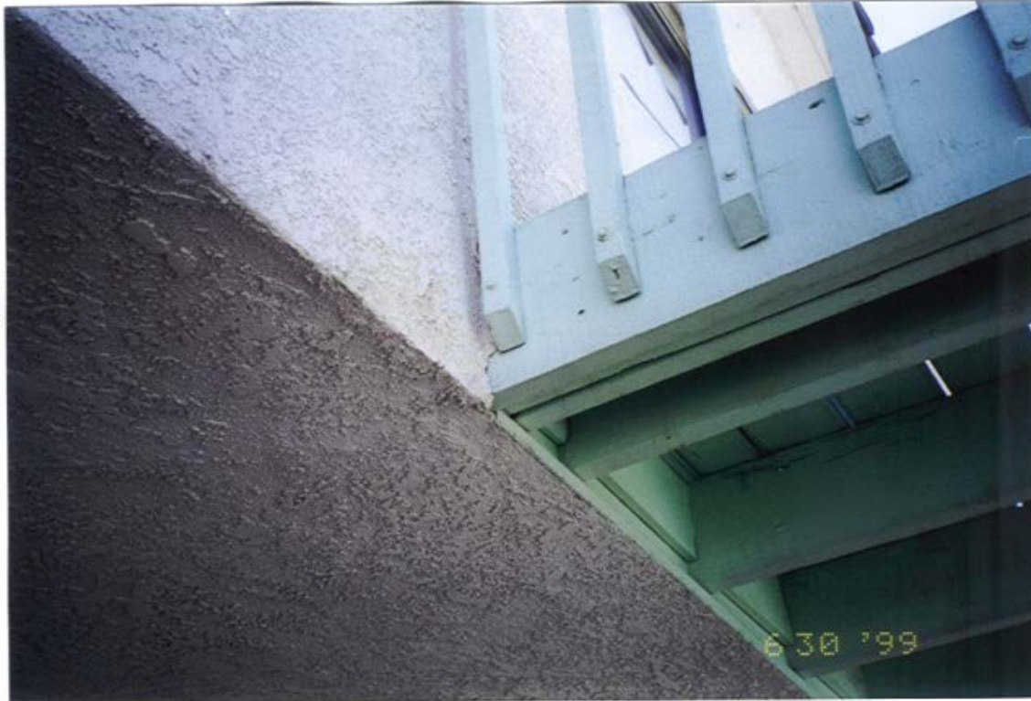
Balcony connection to residence with cracked stucco
