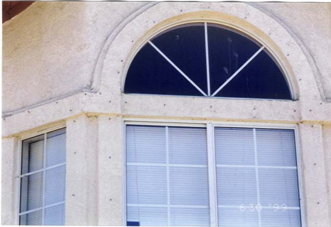
Upstairs window with approximately 100 nails into stucco
