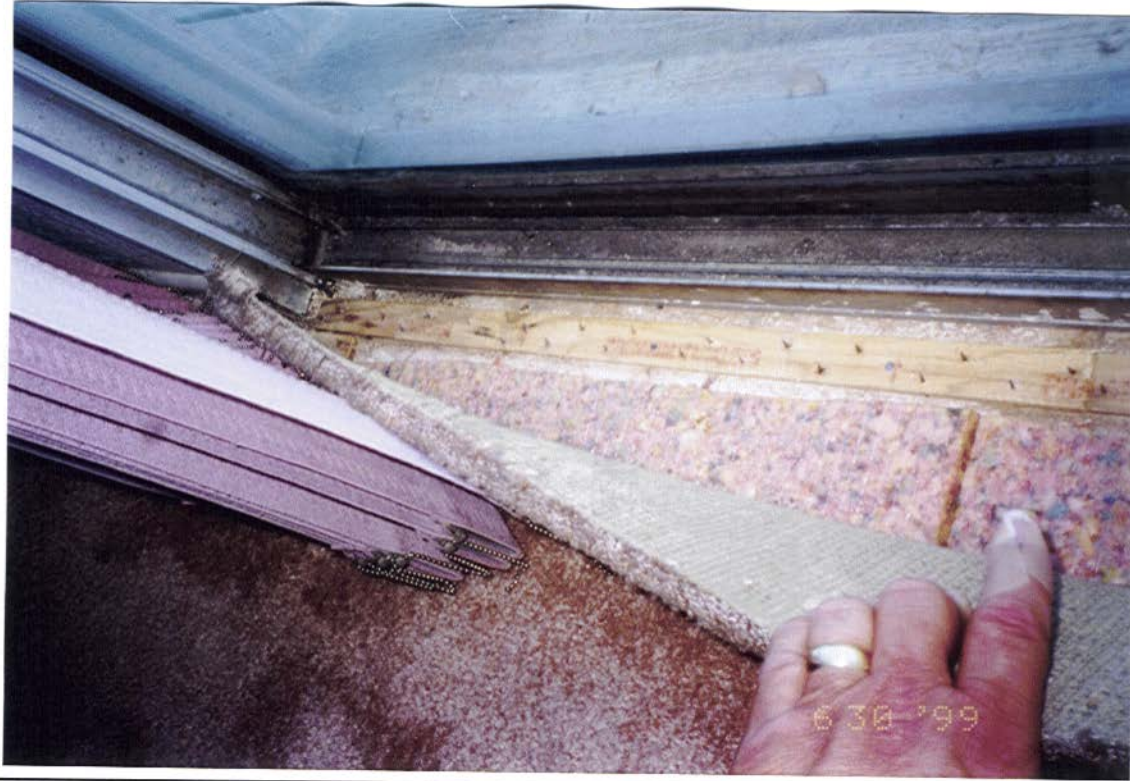
Master bedroom sliding glass door and carpet tack strip closed side (begin of roll #6)
