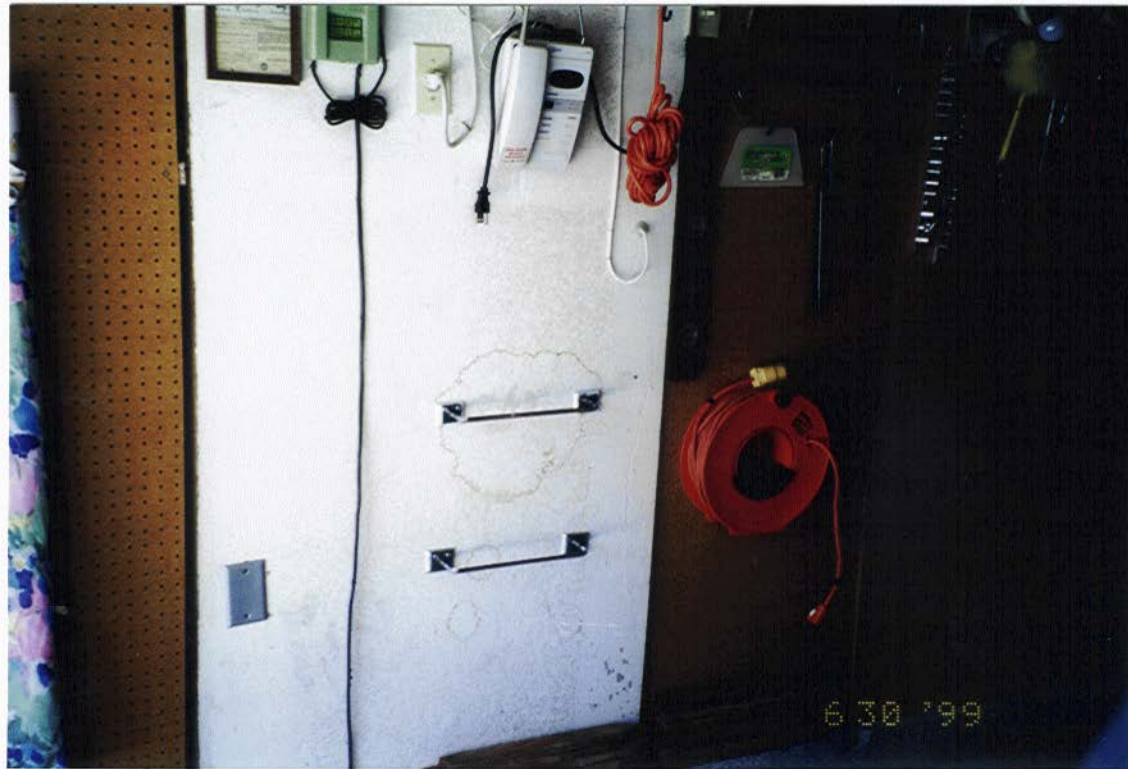
Garage wall water stains on exterior side (opposite front door)
