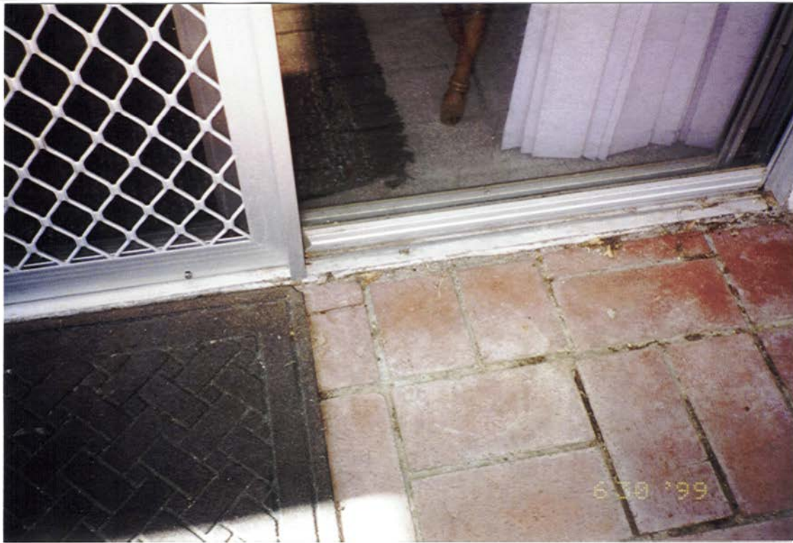
Backyard family room sliding glass door track with hole in track
